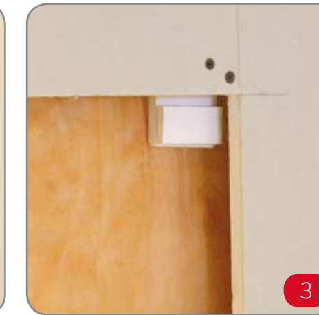
3 Fix installation lugs using two drywall screws secured through the front of the plasterboard into the plastic lug.
