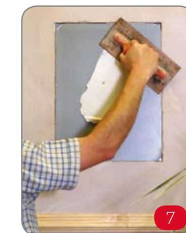
7 For drywall applications only, set panel back 1mm to 2mm from front wall. Fill joint and skim surface with Easi-fill lightweight repair plaster.
